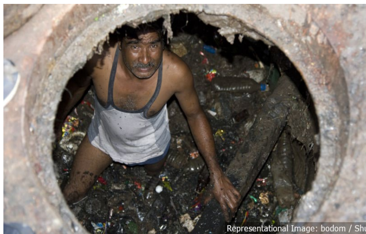
Figure 1-10 Solid waste dumping in the sewer
