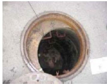
Offset of manhole block
