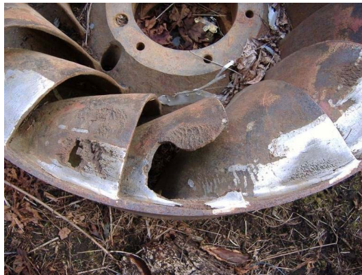
Figure 4-16 Typical cavitation damage of an impeller
