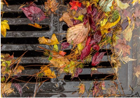
Figure 94: Debris at grating Pic 1
