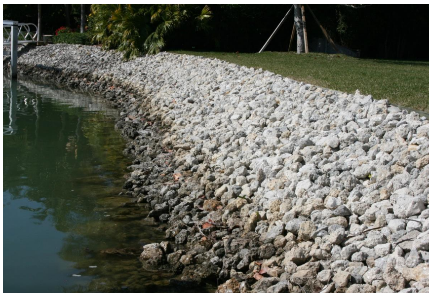
Figure 97: Riprap layer around Banks
