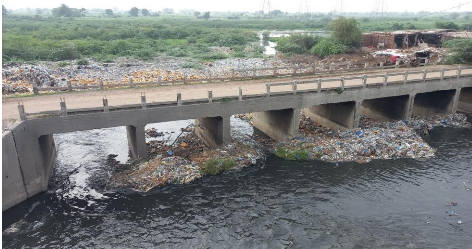
Figure 5-7 Garbage accumulation causing blockage in Drain
