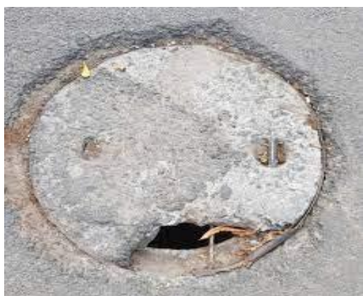
Figure 118: Damaged Manhole Cover
