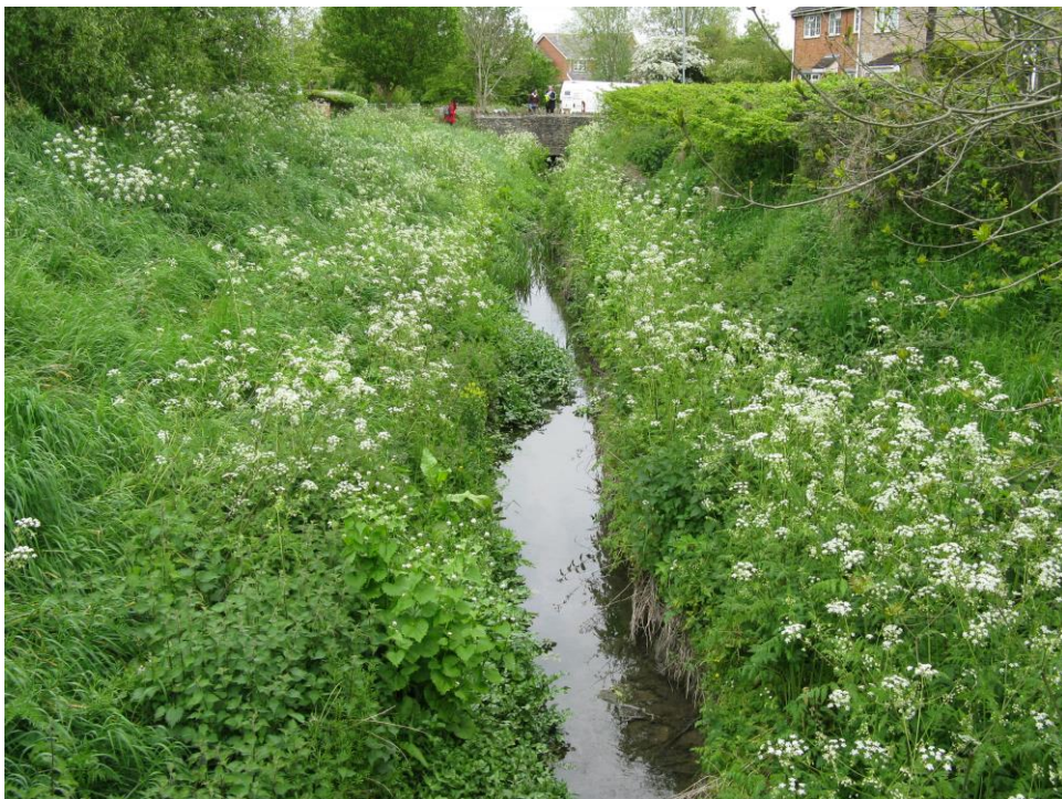
Figure 96: Vegetation at drains
