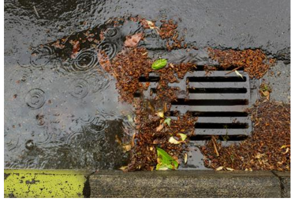
Figure 95: Debris at grating Pic 2
