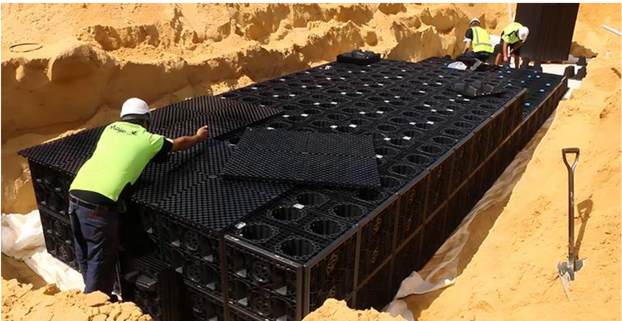
Figure 26: Underground Vaults Tanks
