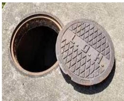
Figure 119: A new Manhole Cover
