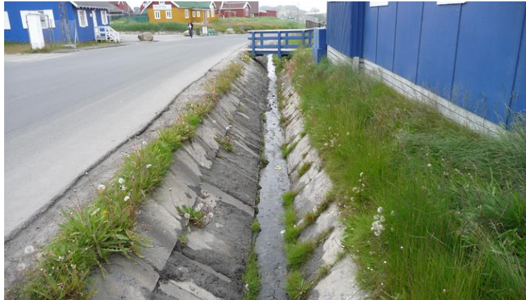
Figure 129: Deep ditches such as this are a safety hazard
