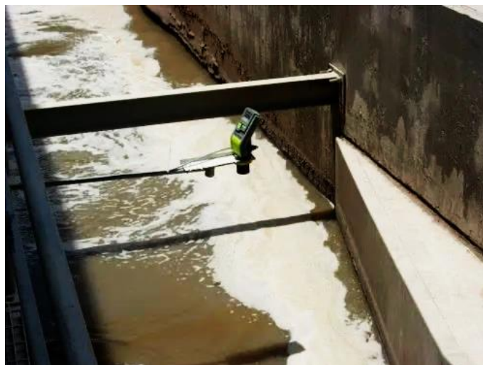
Figure 41: Doppler flow meter installed on a drain
