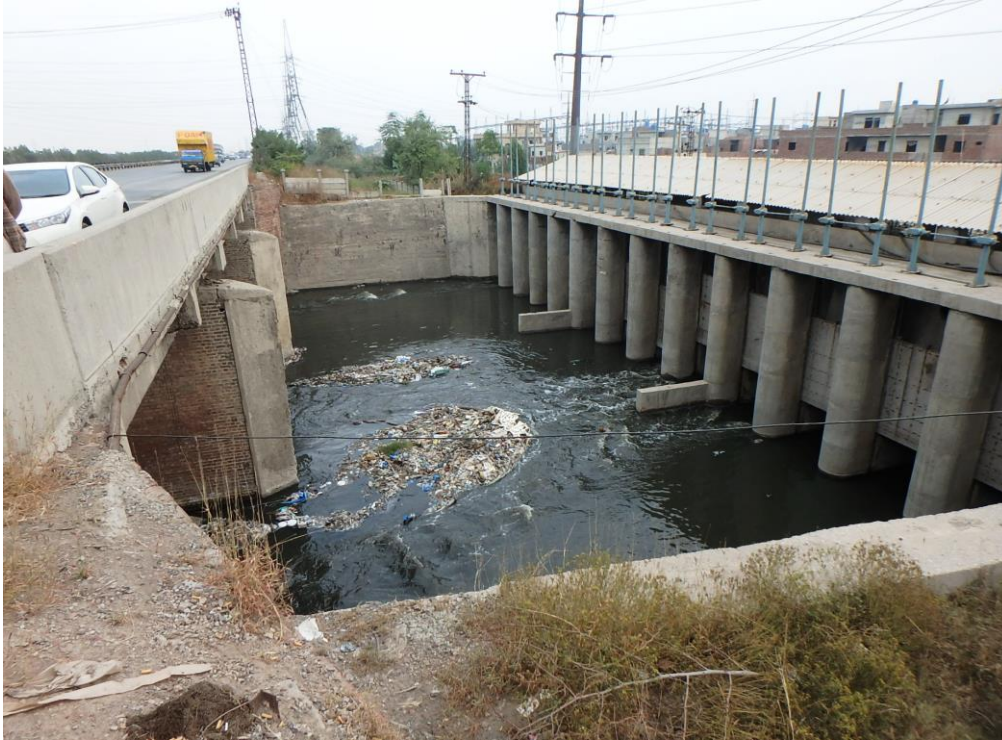
Figure 5: A view of storm water drain regulating structure and Pumping Station
