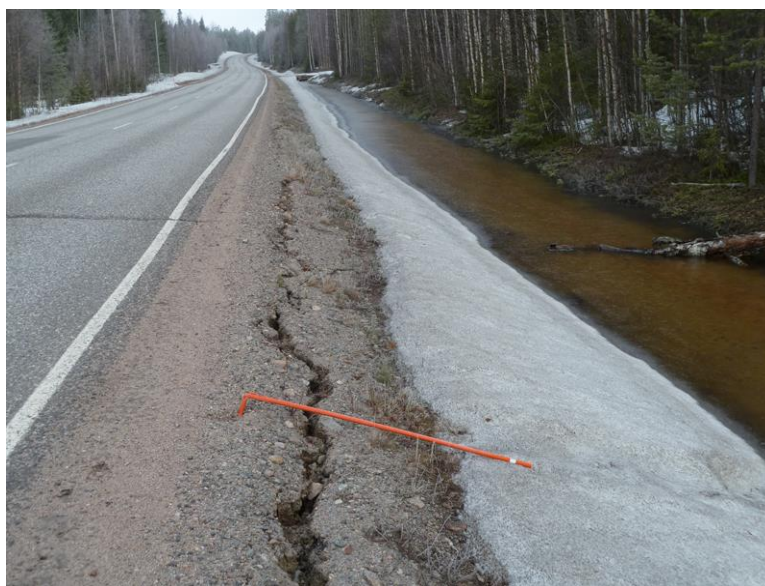
Figure 127: Deterioration of pavement edge and shoulder
