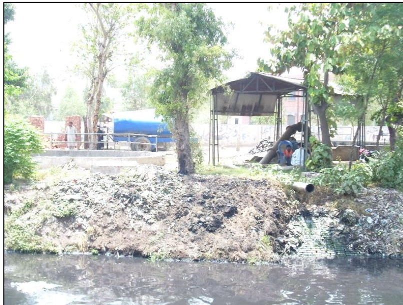
Figure 62: Wastewater lift station discharging into storm drain
