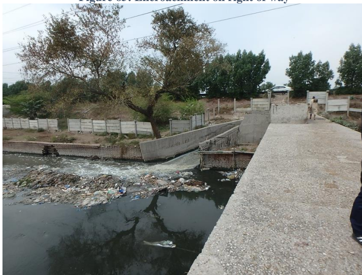
Figure 66: Deteriorated and Damaged Sections of Storm Water Drains
