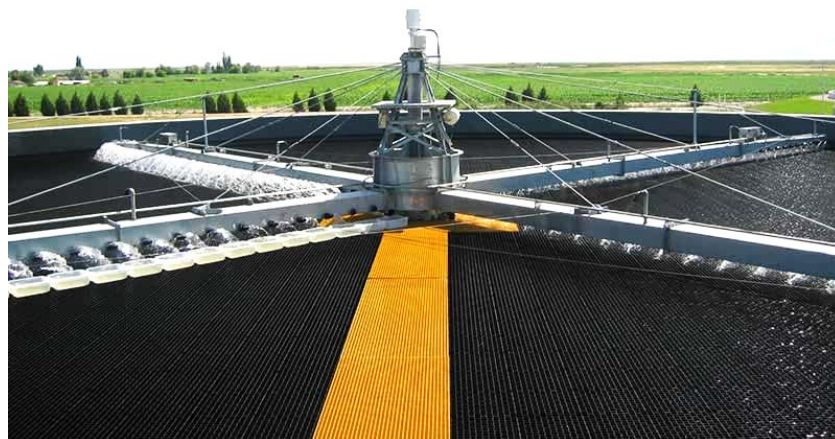
Figure 2-5: Sprinkler of a TF
