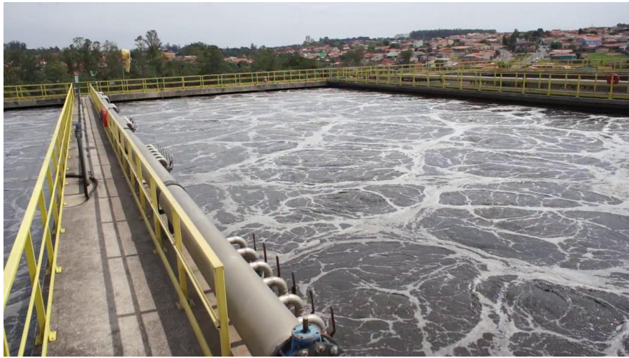
Figure 1-4: Secondary Treatment (Biological Reactor)
