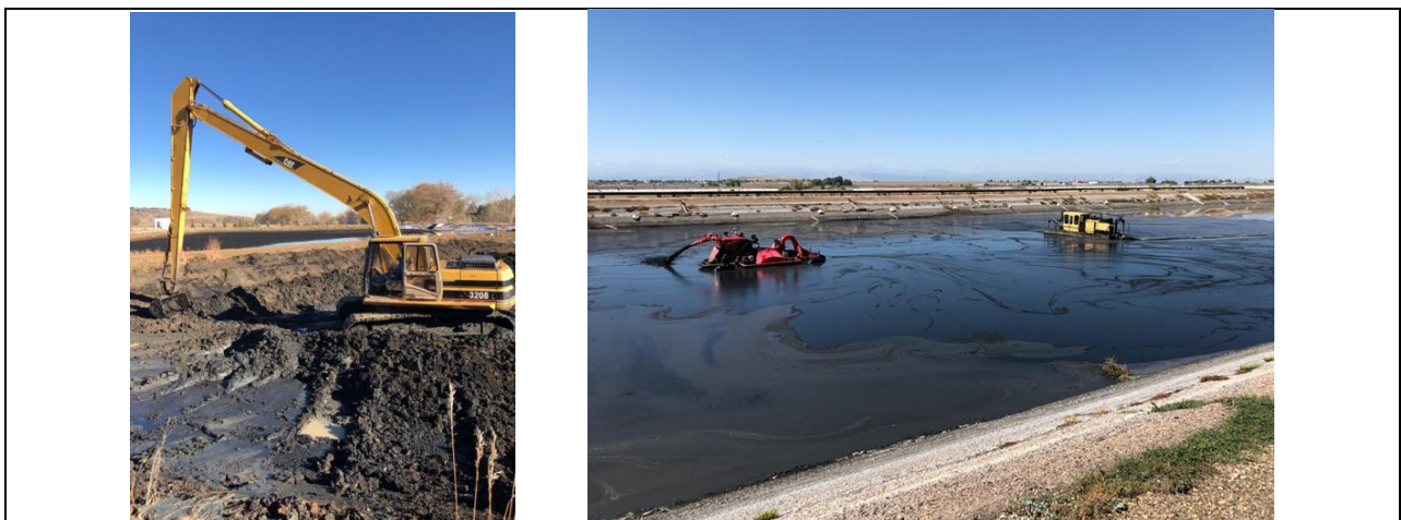
Figure 7-5: Use of pumps
