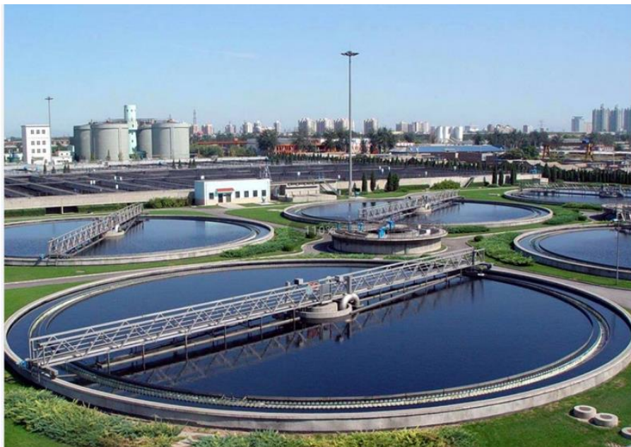
Figure 1-5: Secondary Sedimentation Tank
