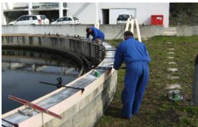
Figure 1-7: O&M of WWTP
