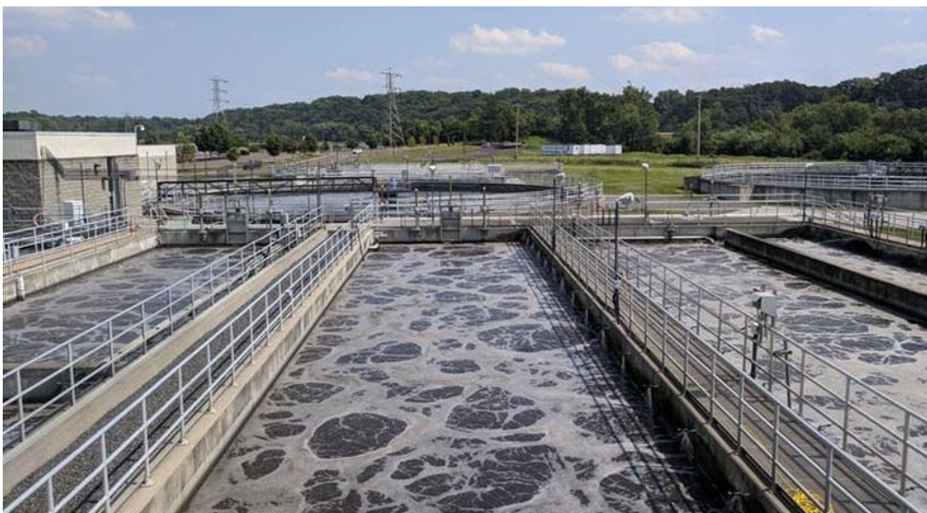
Figure 2-8: Aeration Tank/Biological Reactor
